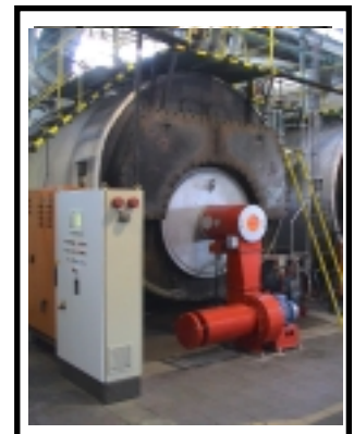
Burner and Electric Panel
