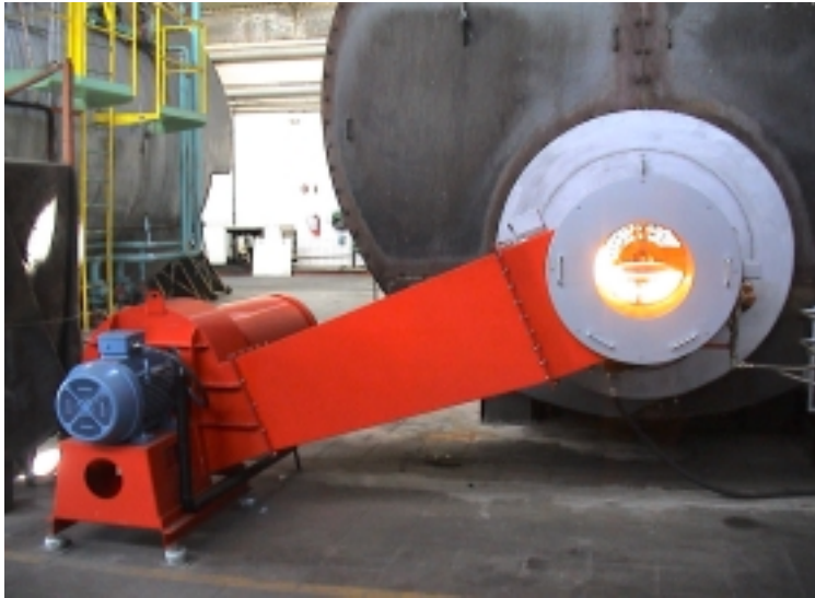
18 Ton Boiler with Limsfield Burner.
