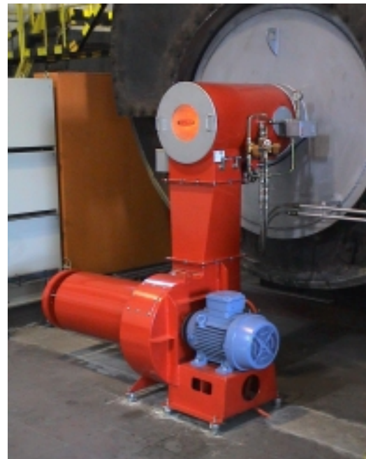
7.2 Ton Boiler with Limsfield Burner
