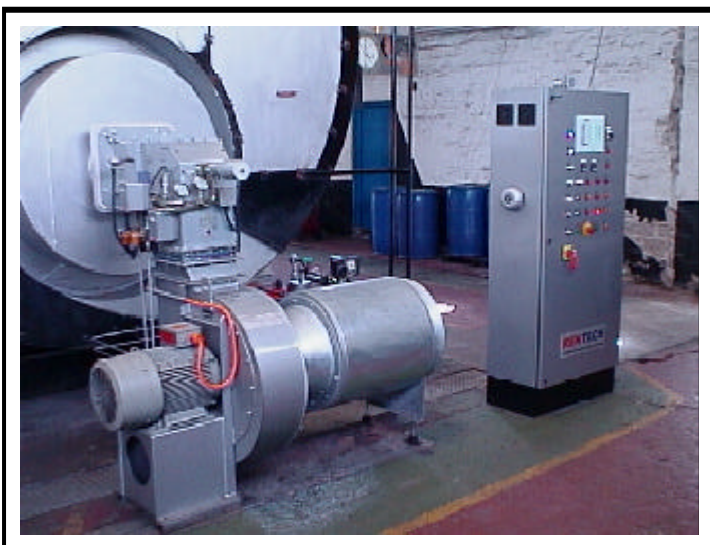
Boiler No.4 Burner and Control Panel
