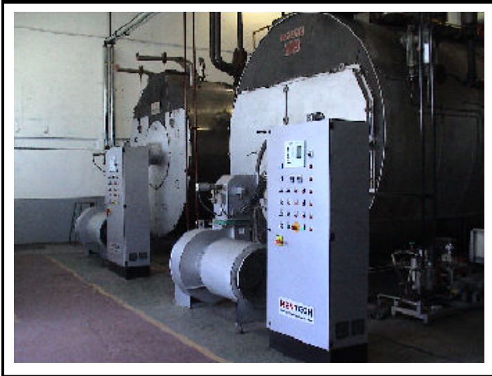
Boilers 1 & 2 with Autoflame and Pressure Jet Burners.
